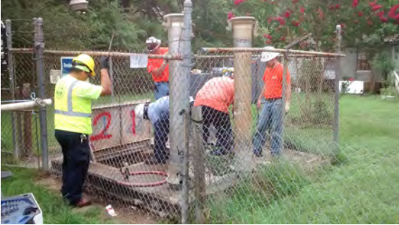
BRECKINRIDGE LIFT STATION Chip Anderson • Dustin Stark • Bobby D'Neal • Syl Causey • Charlie Dukas
