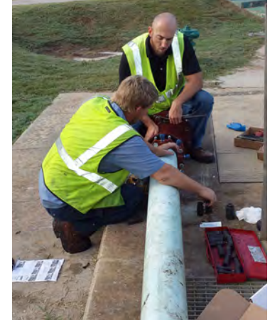
Ben Morrow and Ashley Veal begin installation of suction line to drain the clarifier.
