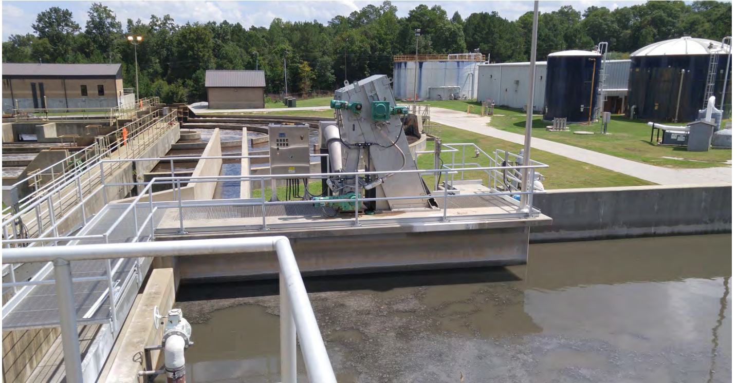
ROCKDALE COUNTY'S NEW WASTE ACTIVATED SLUDGE (WAS) PUMP STATION
