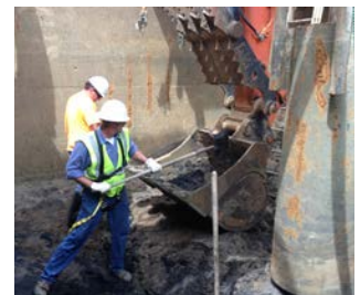
Jerry West and Matt Davis work to remove sand from the WWTP grit system
