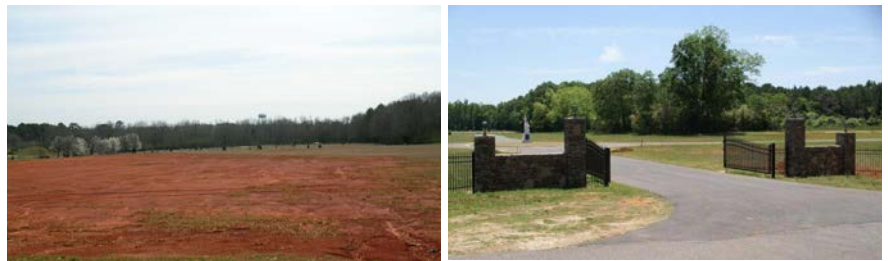
Team Opelika Builds New Section of Evergreen Cemetery in City of Opelika
