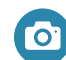
Photo above—New fiberglass wet well structure is lifted and placed over wet well opening
