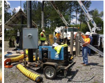
Corporate Safety Director Darrel West helps to insure the Southwest Lift Station repair is safe, efficient and effective
