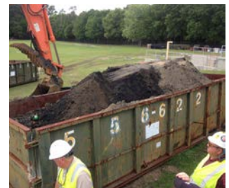
Tommy Coker and Don Pate (foreground) coordinate the effort to remove over 30 cubic yards of material from the grit system
