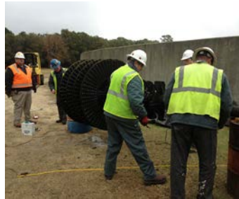
Mickey Roberts, Joey Stevenson, Jeff Buchanan and Jerry West repair one of the aerator sections
