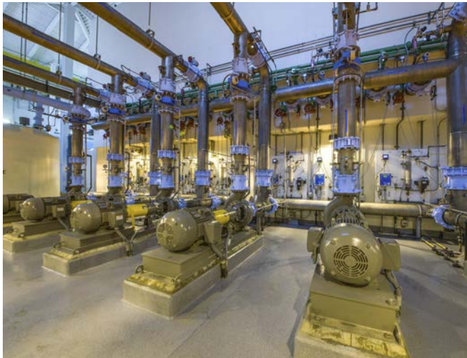
Forsyth County's New Membrane Plant
