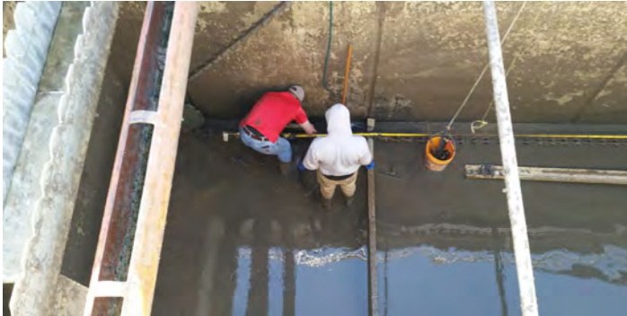
CLARIFIER AT WINDERMERE
