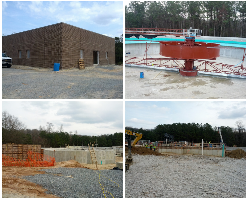
ESG Engineering is assisting Team Warner Robins in the upgrades to the Wastewater Treatment Plant Top row, left to right: Administration Building and new Clarifiers. Bottom row: Headworks and RAS/WAS Effluent Pump Station
