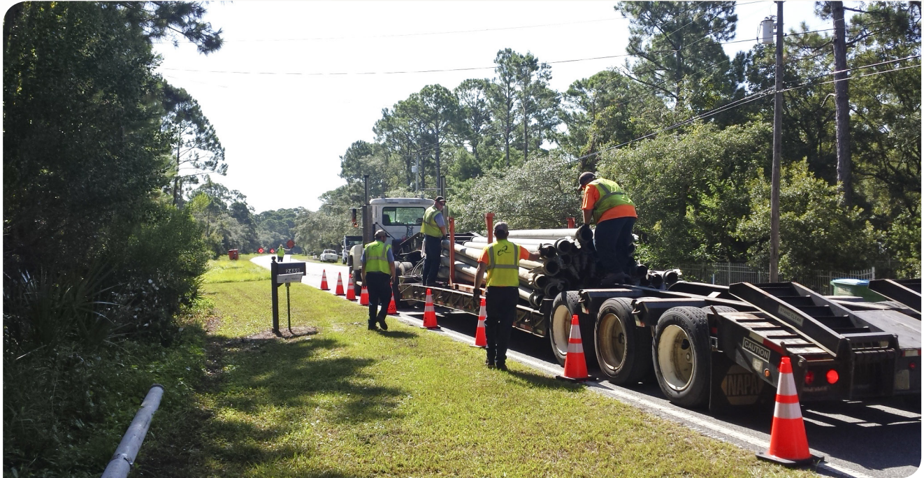
By-pass Piping | Wakulla County Road and Bridge crew assists C&D crew with by-pass piping
