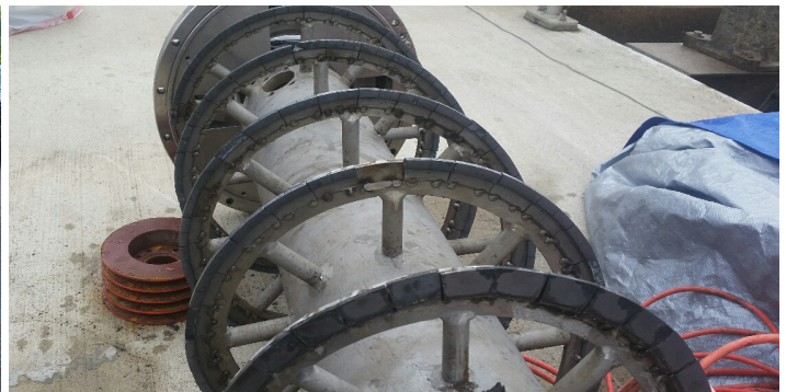
Scroll conveyor from The Manor WRF centrifuge removed from the bowl assembly
