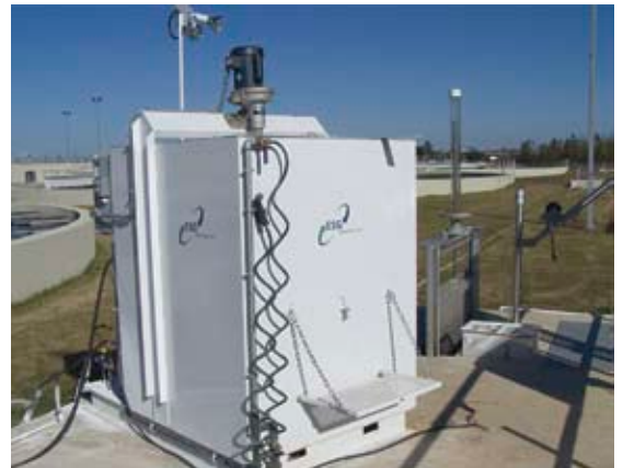
New Polymer and Lime Pumping System
