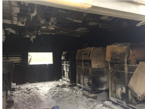
James Creek WRF Blower Room Fire
