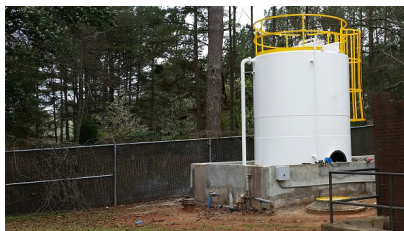
New Lime Tank/Water Plant
