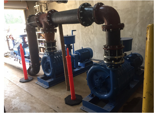
Temporary Blowers for James Creek WRF
