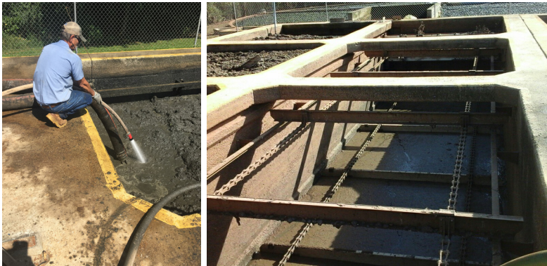
Dwight Smith cleaning primary clarifiers
