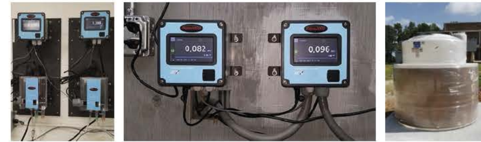
1 New Chlorine Analyzers 2 New Filter Turbidimeters 3 New Fluoride Feed System 4 New Motor Install for Sludge Mixer
