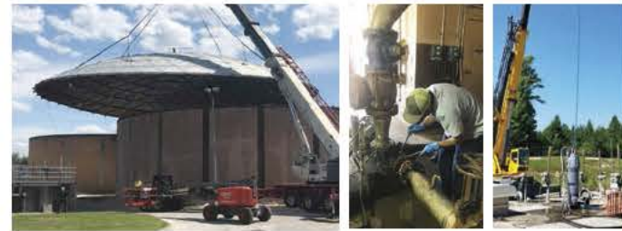
1 Digester 1 Top Removal 2 Fernando Cruz WAS Pump Derag 3 Spirit Creek Flygt LS pump installation
