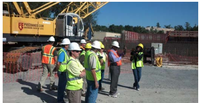
Warner Robins Mayor Chuck Shaheen and members of the City Council on site to review the progress of the Sandy Run WWTP upgrade
