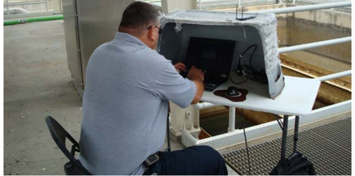
Bryan Cloud backwashing filter using laptop
