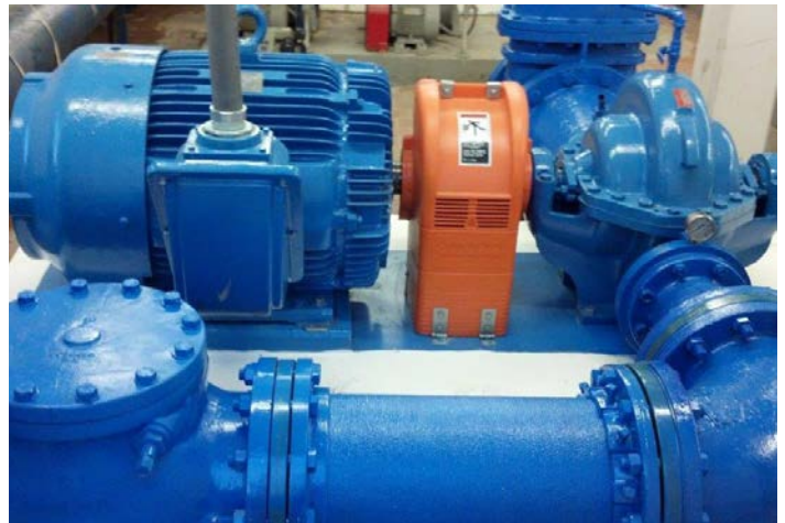
New High Service Pump at Water Plant #1
