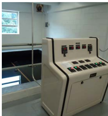
Rehabilitated Filter with New Console
