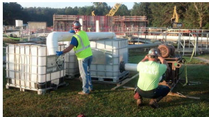
Kelly Jarriel and Chip Anderson installing the Moyno pumps at Sandy Run Wastewater Treatment Plant
