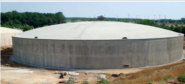
The New 8 Million Gallon Clearwell
