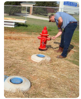
Ryan Bode , Line Maintenance Supervisor, installs new water main at new facility.
