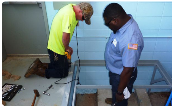
Our new NPDES permit for backwashing filters at the water plants will require us to dechlorinate prior to discharging. City and ESG personnel combined forces to fabricate chemical feed system. Ben Carter (left) and Antwann Fann (right) are shown installing the system. Completing the work in-house saved the City thousands of dollars on installation.
