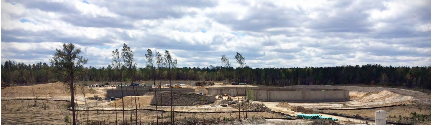
NEW FACILITY SPEARS CREEK INTERMITTENT CYCLE EXTENDED AERATION-SANITAIRE (ICEAS)
