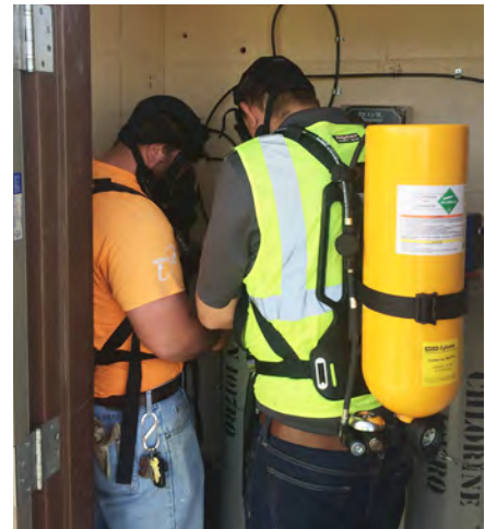
Brian Rowland and Zac Conlon installing the first set of Cl2 tanks at the Northeast Well in Moultrie
