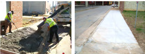
SIDEWALK REPLACEMENT — Allen Johnson, Dale Cook, Aaron Grant and David Petty removed the broken sidewalk, poured and screed the new concrete on South 10th Street in Opelika.
