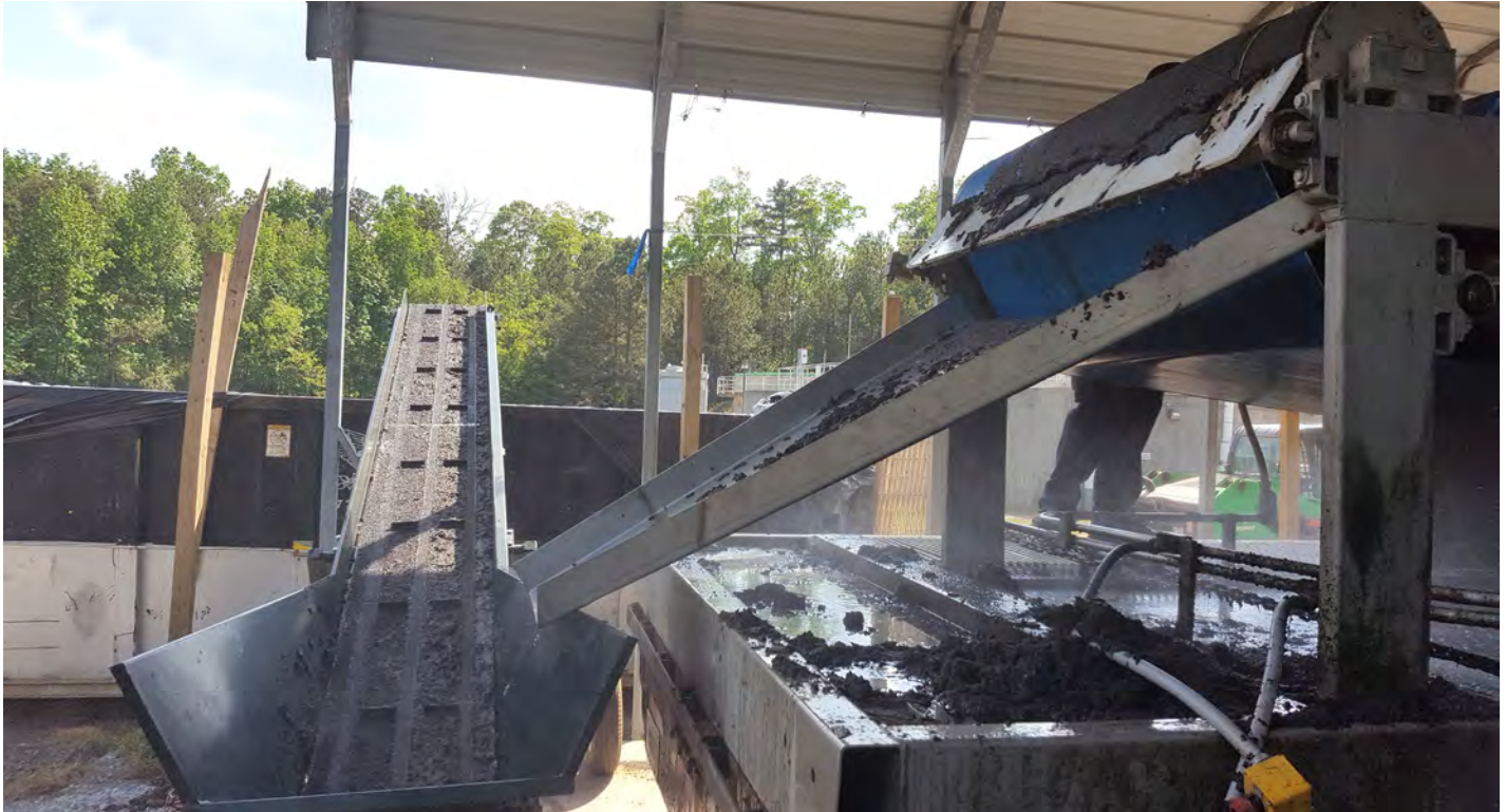
Forsyth County's Dicks Creek Water Reclamation Facility Belt Press
