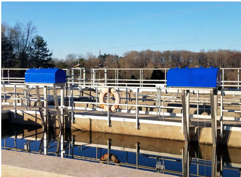
New TRAC-VAC® System at Commerce's Water Plant
