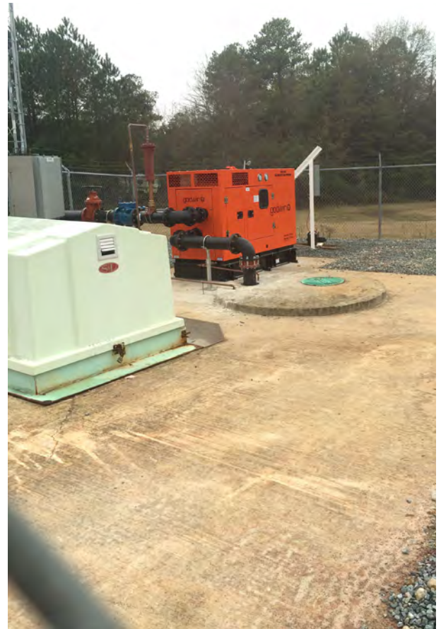
NEW PUMP STATION Lemley’s Pump Station Bypass Pump Upgrade
