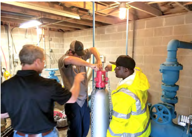
Corporate Safety Director Darrel West provides critical safety training on chlorine cylinders and protocols to Team Hinesville Water operations staff
