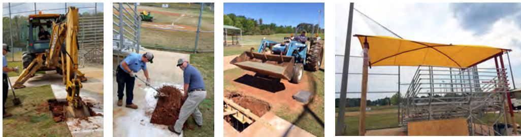
INSTALLATION OF NEW SUN SHADES AT THE MIRACLE FIELD — Ross Coxwell, Derick Reap, Mike McDonald, Rodney Renfroe and Calvin Wallace of Building Maintenance and Bruce Boyd of Park Maintenance recently installed two sun shades for the Billy Hitchcock Miracle Field at West Ridge Park. ESG played a vital role in helping to bring the Miracle Field to the City of Opelika in 2007. The Miracle Field is not only a baseball field, but includes an entire environment suited for special needs children and adults.
