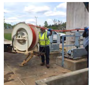
Mickey Thompson rodding the grit valve at the Westside Wastewater Treatment Facility. Mickey helps keep our wastewater system in perfect working order.
