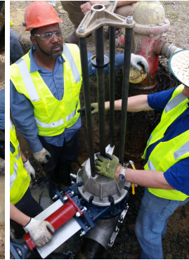
C&D Crew - Albert Collins
