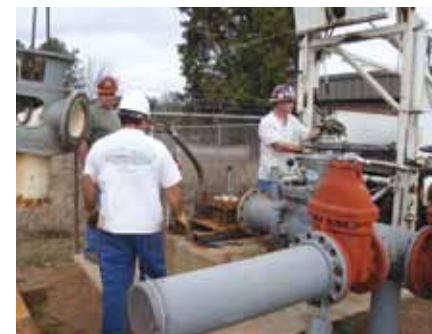
Well 3 • The City of Perry's largest producing well which was repaired and rebuilt by Team Perry
