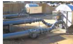
Left: Effluent filters before Right: Effluent filters after
